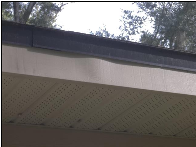
2.5 Item 1(Picture) Fascia is Bent
