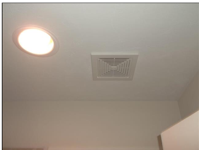
9.4 Item 3(Picture) Bathroom Vents
