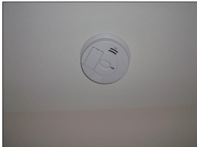
7.7 Item 1(Picture) Smoke Detectors
