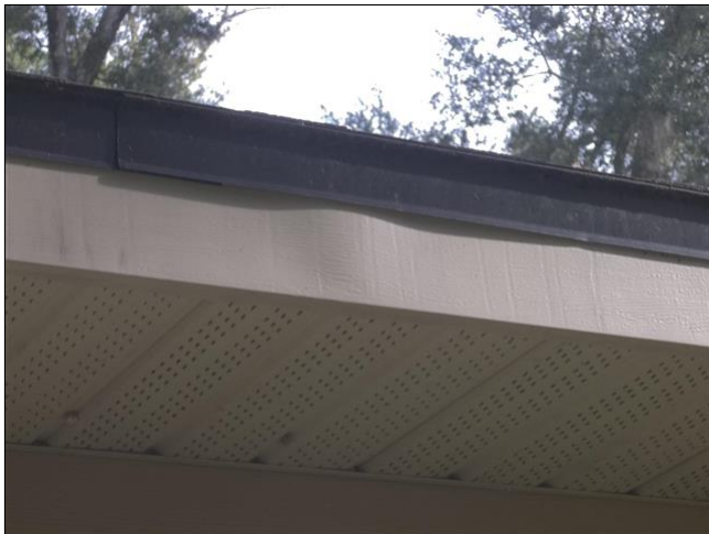
2.5 Item 1(Picture) Fascia is Bent
