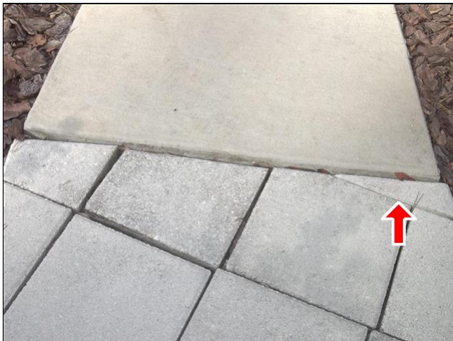
2.3 Item 3(Picture) Potential Tripping Hazard
