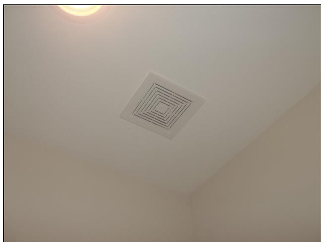
9.4 Item 1(Picture) Bathroom Vents
