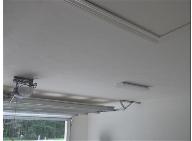
3.0 Item 2(Picture) Garage Ceiling
