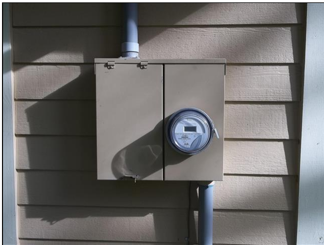
7.0 Item 1(Picture) Meter and Service Entrance
