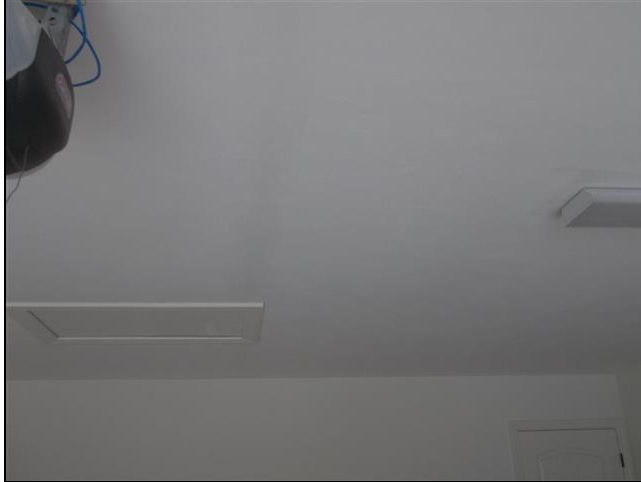
3.0 Item 1(Picture) Garage Ceiling
