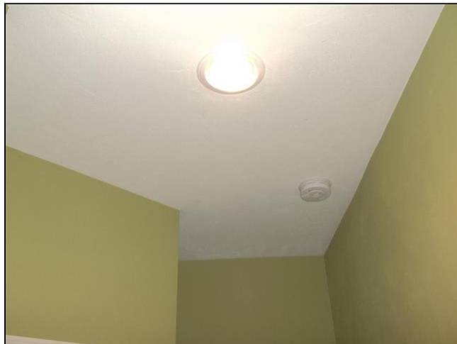
4.0 Item 3(Picture) Ceilings
