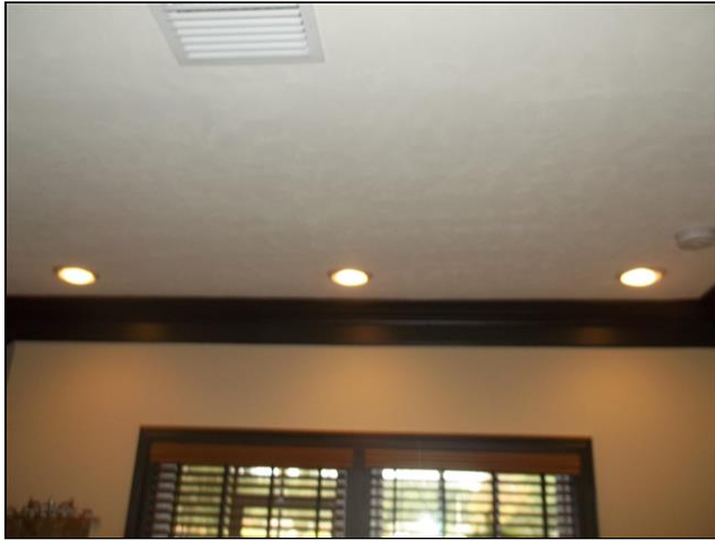
7.3 Item 1(Picture) Lighting
