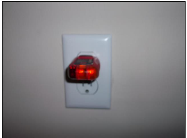
7.4 Item 2(Picture) Receptacles
