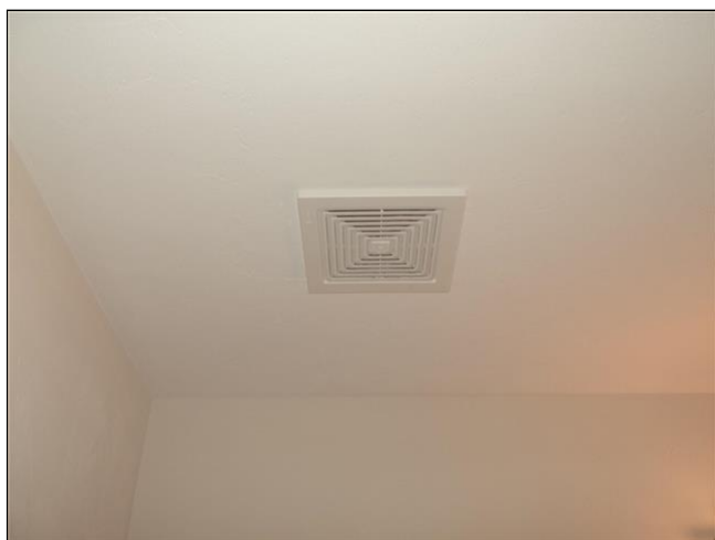
9.4 Item 2(Picture) Bathroom Vents
