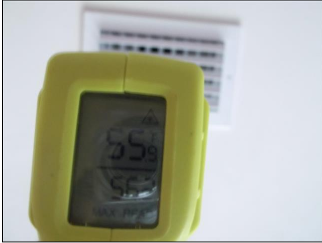
8.6 Item 1(Picture) Cooling Sources
