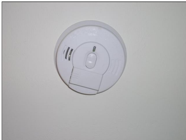
7.7 Item 2(Picture) Smoke Detectors
