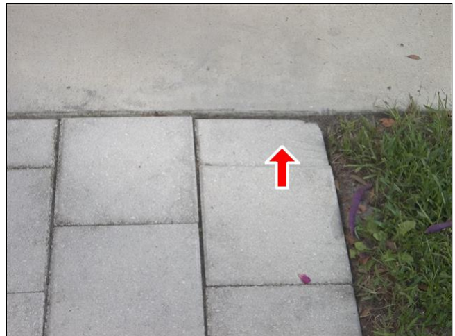
2.3 Item 4(Picture) Potential Tripping Hazard
