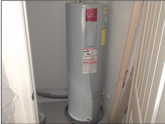
6.2 Item 1(Picture) Water Heater
