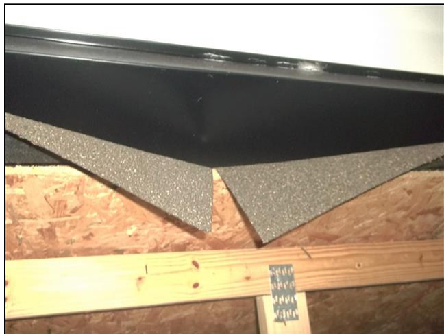
9.3 Item 1(Picture) Roof Vent
