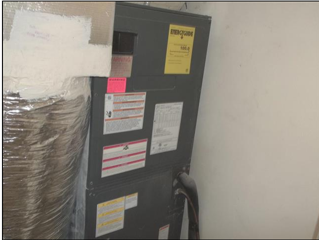
8.4 Item 1(Picture) Air Handler
