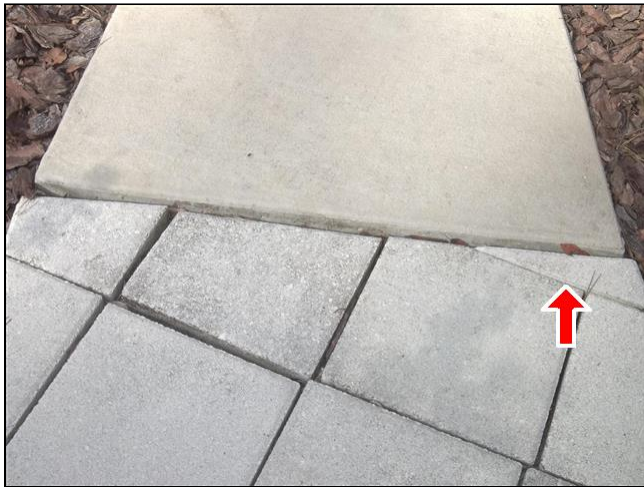
2.3 Item 3(Picture) Potential Tripping Hazard
