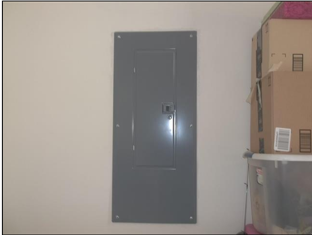
7.1 Item 1(Picture) Main Panel
