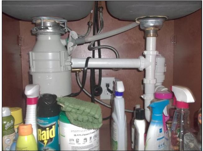
6.1 Item 2(Picture) Kitchen Sink Plumbing
