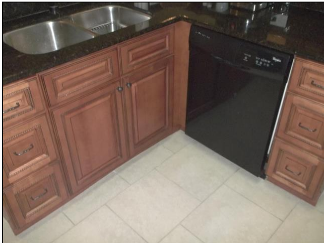
4.4 Item 3(Picture) Cabinets
