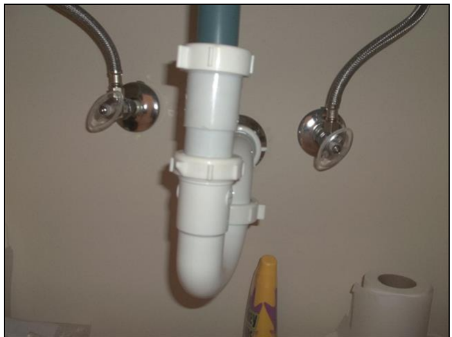
6.1 Item 4(Picture) Bathroom Sink Plumbing
