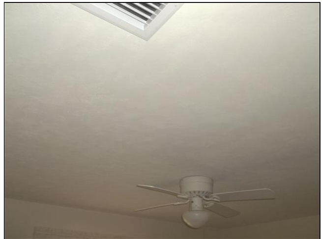
4.0 Item 2(Picture) Ceilings
