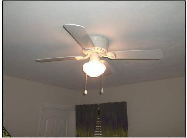
7.3 Item 2(Picture) Lighting
