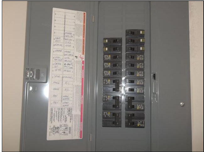
7.1 Item 2(Picture) Main Panel
