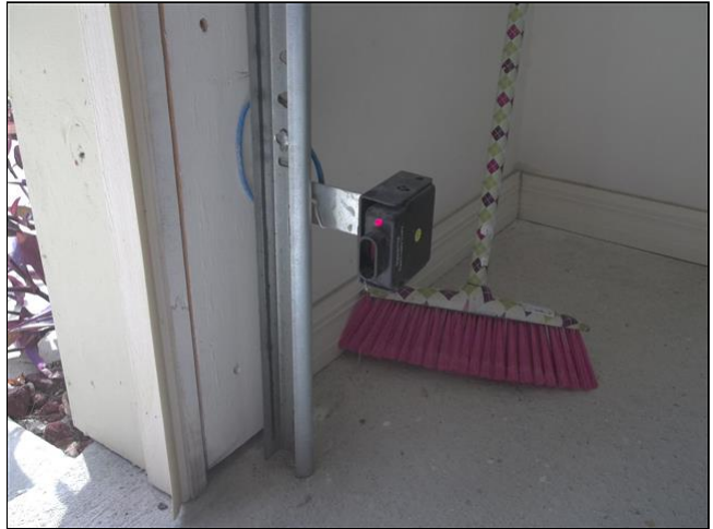
3.5 Item 2(Picture) Garage Door Sensors
