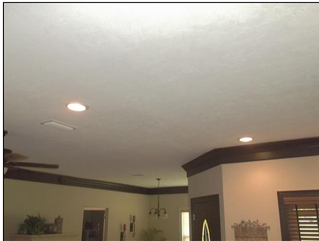
4.0 Item 1(Picture) Ceilings
