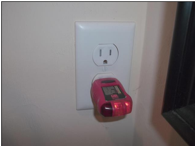
7.4 Item 1(Picture) Receptacles
