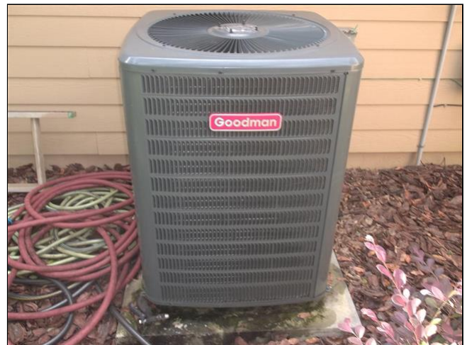
8.4 Item 4(Picture) Outside AC Unit
