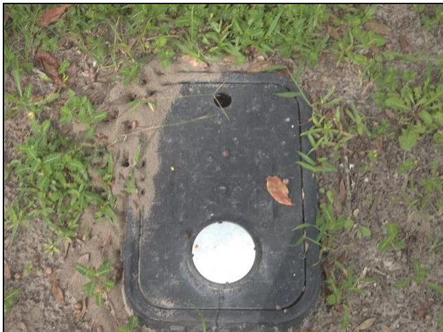
6.3 Item 1(Picture) Main Water Shut Off
