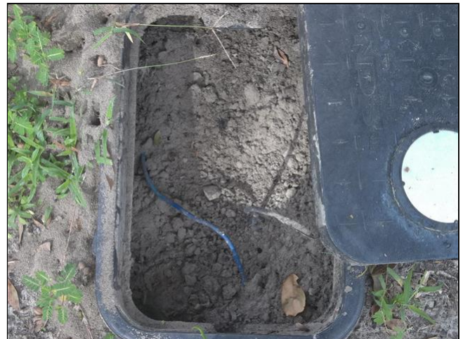
6.3 Item 2(Picture) Main Water Shut Off
