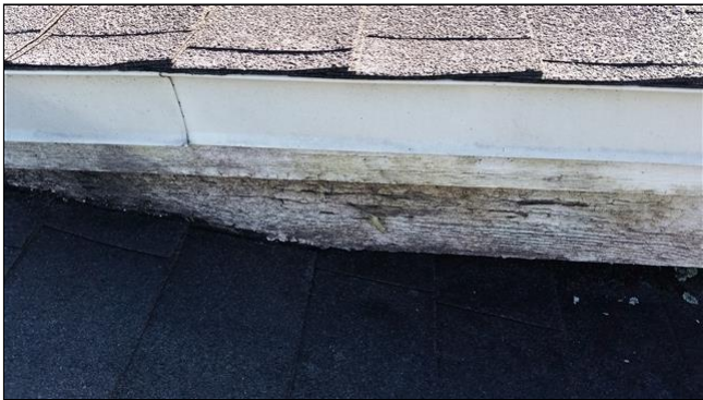
2.5 Item 4(Picture) Worn Fascias
