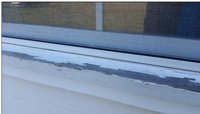
2.2 Item 2(Picture) Worn Trim
