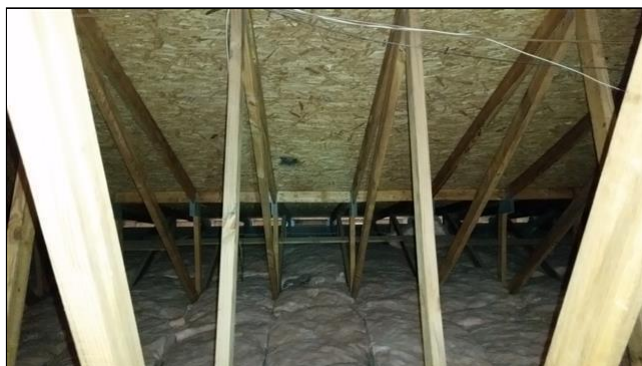
5.4 Item 2(Picture) Moisture Intrusion
