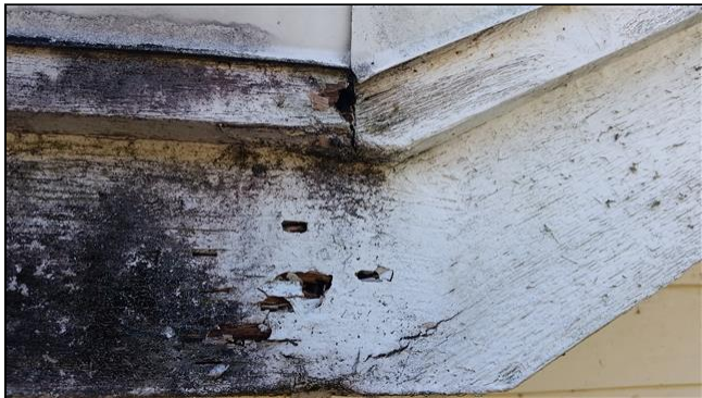
2.5 Item 1(Picture) Wood Rot
