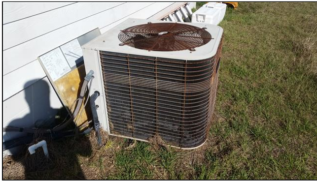
8.8 Item 1(Picture) Condensing Unit
