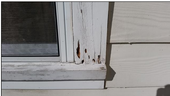
2.2 Item 3(Picture) Wood Rot
