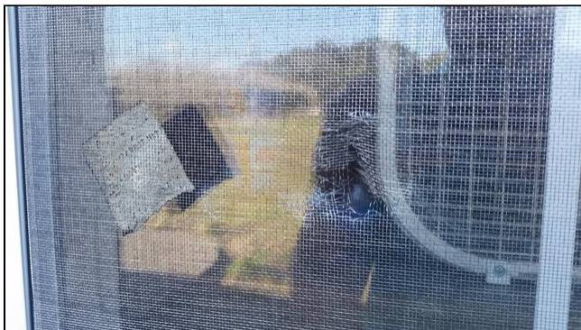
2.2 Item 1(Picture) Damaged Screen
