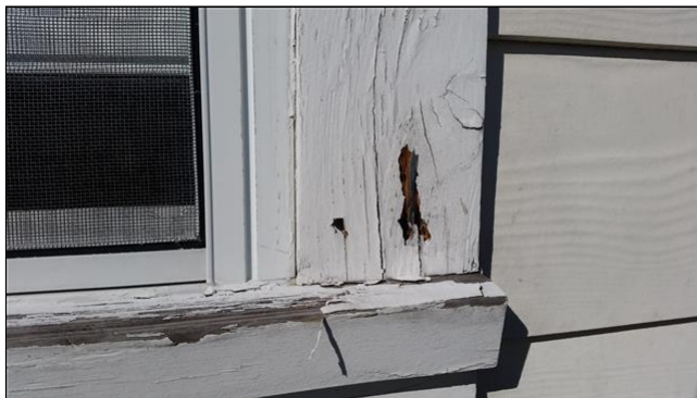
2.2 Item 4(Picture) Wood Rot
