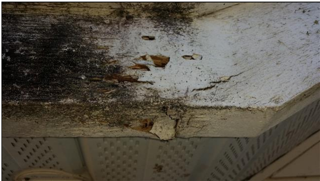
2.5 Item 2(Picture) Wood Rot
