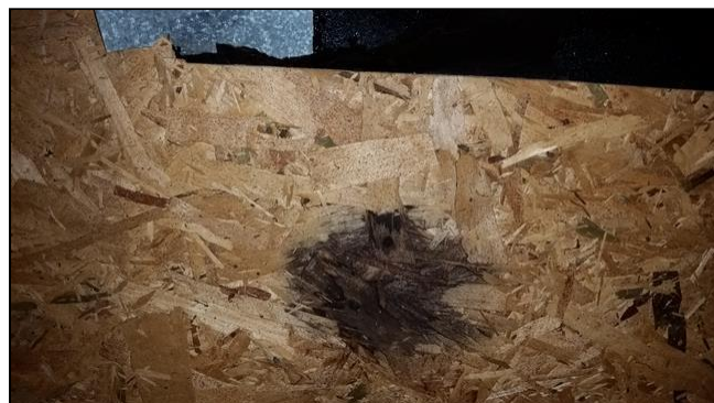
5.4 Item 1(Picture) Moisture Intrusion
