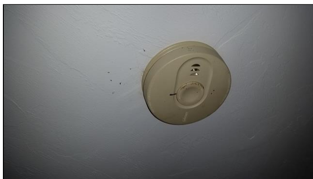
7.7 Item 1(Picture) Smoke Detector
