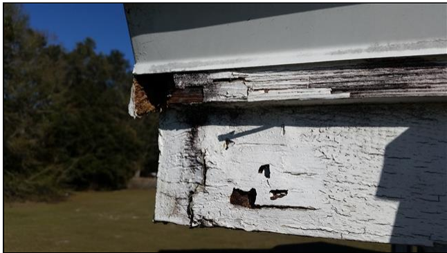
2.5 Item 3(Picture) Wood Rot
