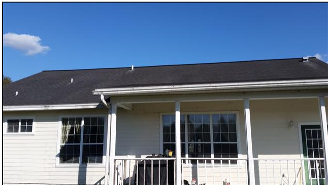
2.5 Item 5(Picture) Loose Fastener
